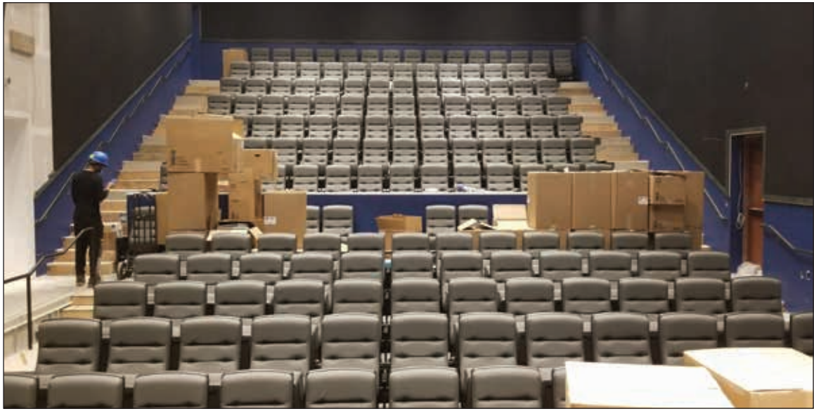
Doylestown's County Theater is nearing completion of its expansion and renovation project. The interior of the existing two theaters have new, larger seating with more leg room.
